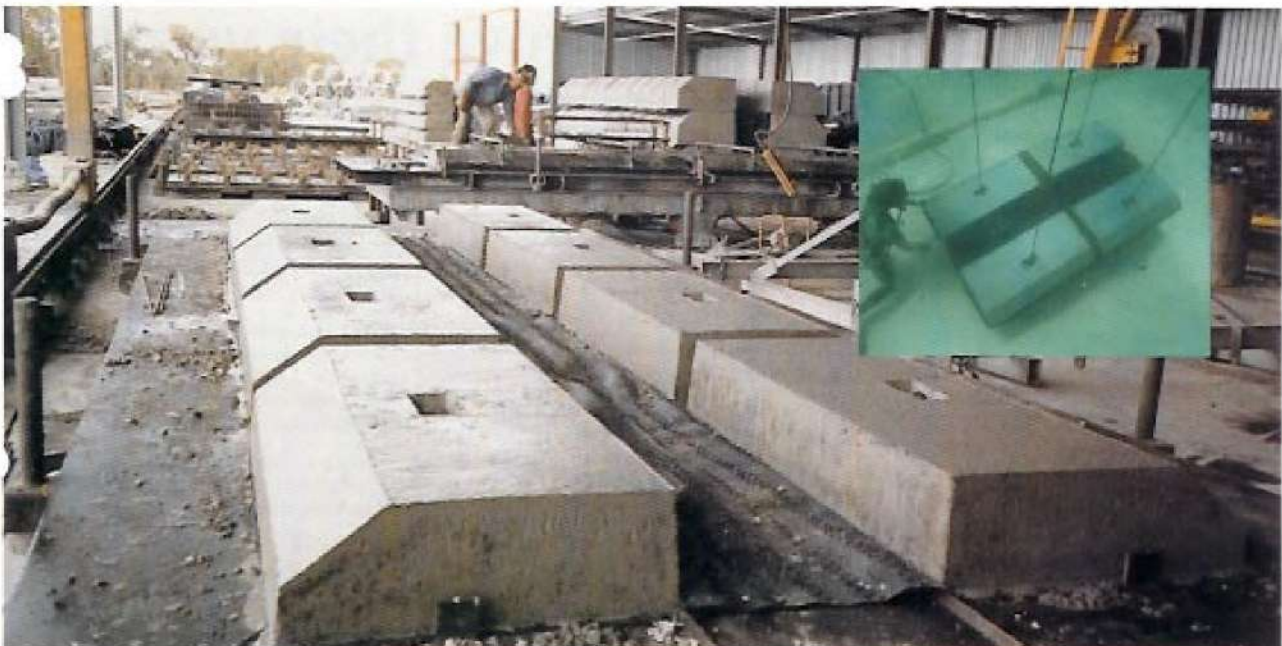
Inset below: A diver positions the Flexmat ready for lowering onto the pipeline seen in the top left of the picture.
